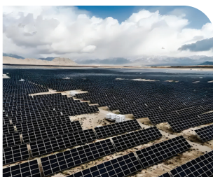
Solar power plant
